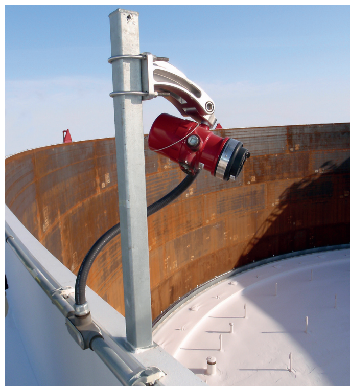
Optical flame detectors can be pole mounted for open roof floating tanks
